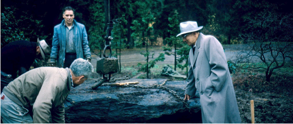
Portland Japanese Garden's original designer, Professor Takuma Tono, supervises the construction of the Flat Garden. 📷 William "Robbie" Robinson
